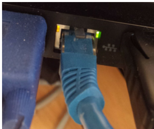
Figure 24: Ethernet LEDs blinking
