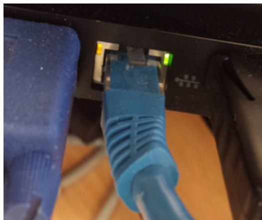
Figure 25: Ethernet LEDs blinking
