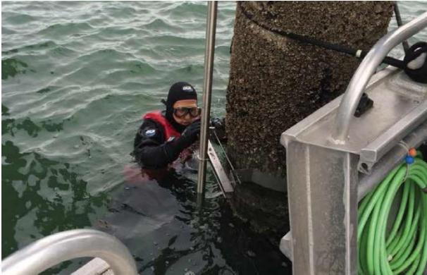
Figure 5 Photo of diver during installation procedure. The specially-designed (green) online cable can be seen coiled up in the bottom right.
